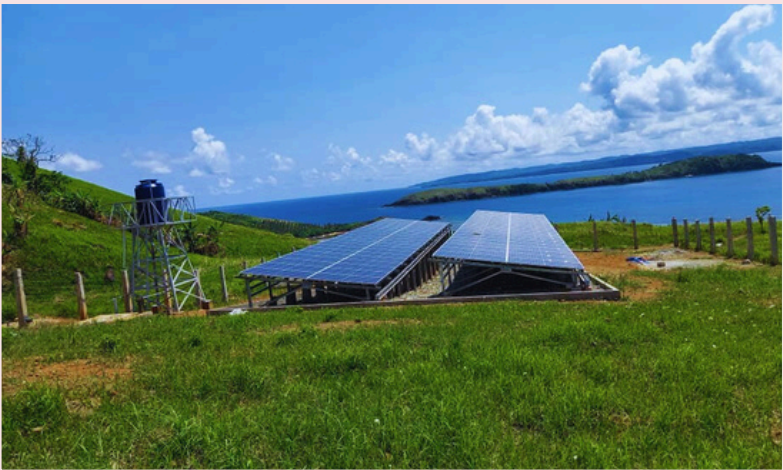
Palumbanes Solar PV with ESS
