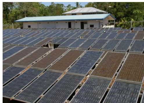
The 28-kW peak centralized PV system in Pangan-an Island was installed through Belgian assistance (photo courtesy of IICA)
